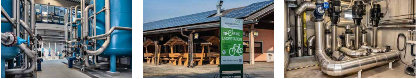
From L to R: critical infrastructure (water supply), photovoltaic e-bike charging station, power-to-heat equipment at biomass heating plant, photos: act4.energy
